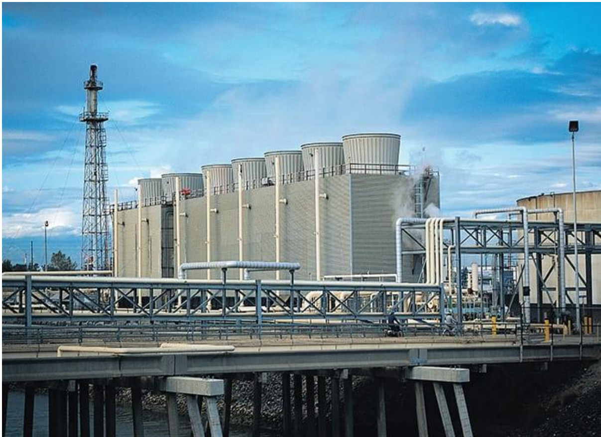
Figure 1. Microbial control must be considered for cooling tower systems to maintain operational efficiency
