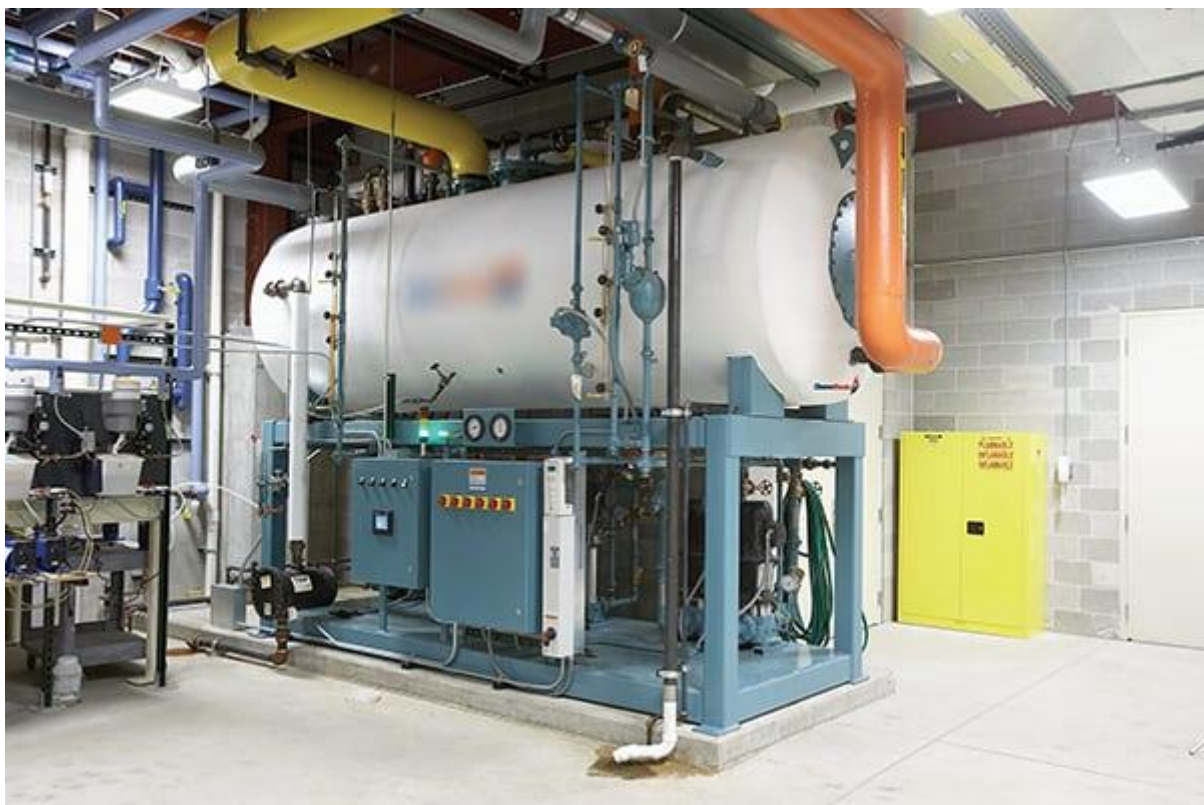
Figure 2. Tray-type de-aerators are designed to remove oxygen from boiler feedwater to avoid corrosion issues
